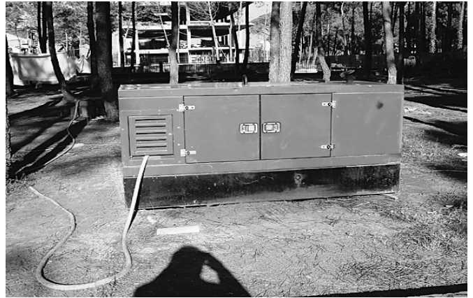
Albania still lacks a solid supply of electricity. Two of these 25KW machines were employed to keep the ZA1A contest station producing on all six bands, without interruption.
